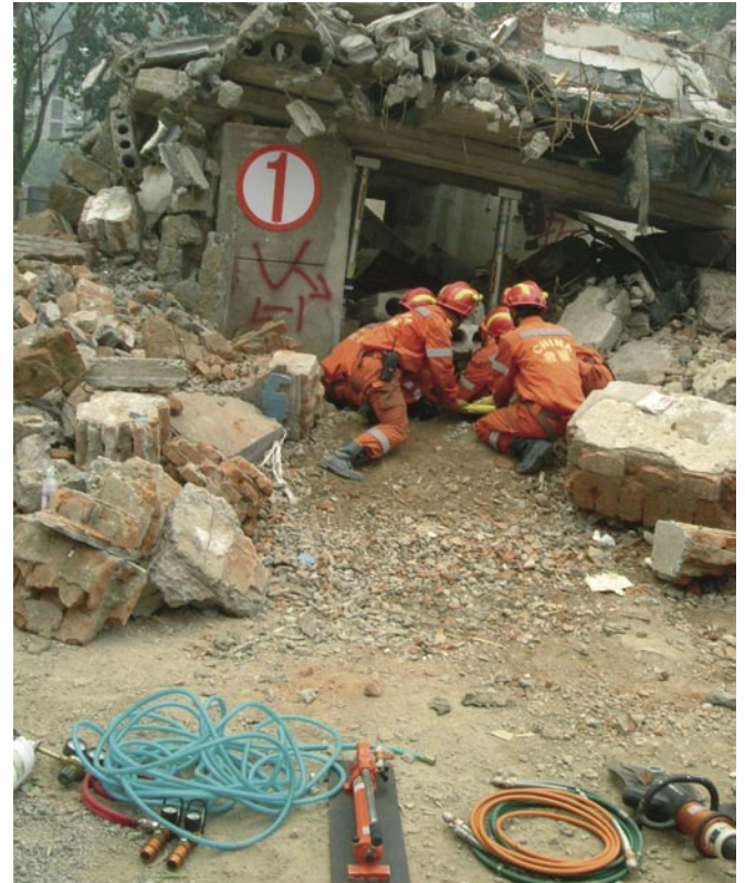
Shoring can provide initial stabilisation where fully braced systems are to be constructed later
